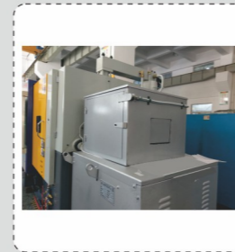
Furnace safety guard
