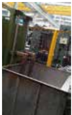
Water cooling device
